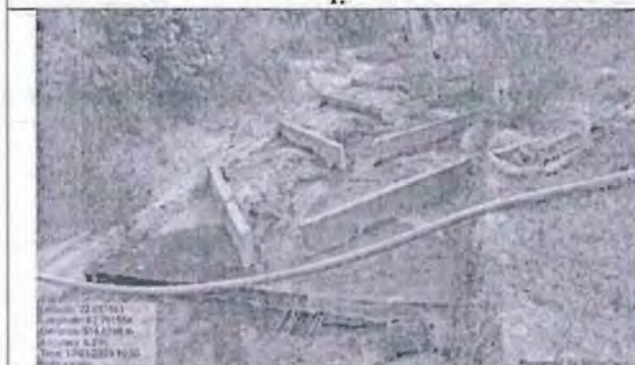
Fig.5. View of one of the settling tank.
